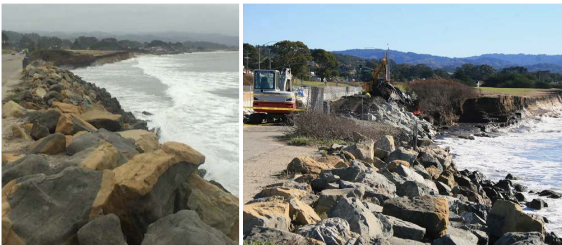
Figure 4.9. Two views of the eroding portions of Surfer’s Beach. Left: View in Summer 2015 from the toe of the east breakwater looking south at the erosion threatening Highway 1. (Photo: Max Delaney) Right: Construction of temporary armoring during winter 2015. (Photo: California Department of Transportation)
